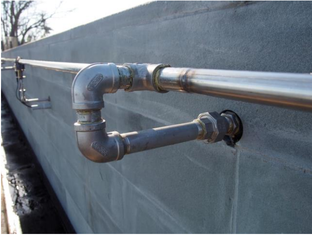
Close up of Main Burner Gas Connection
