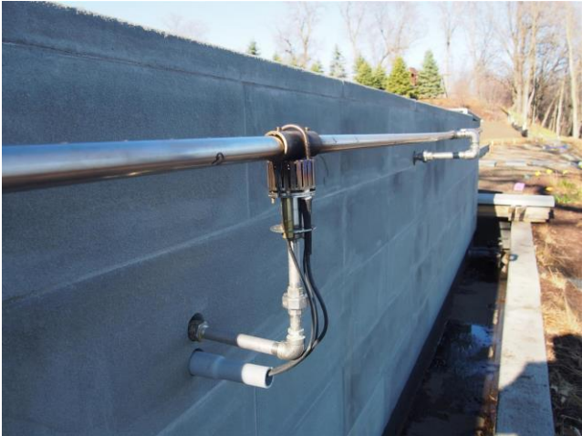
Close Up of Pilot Burner supported by Main Burner
